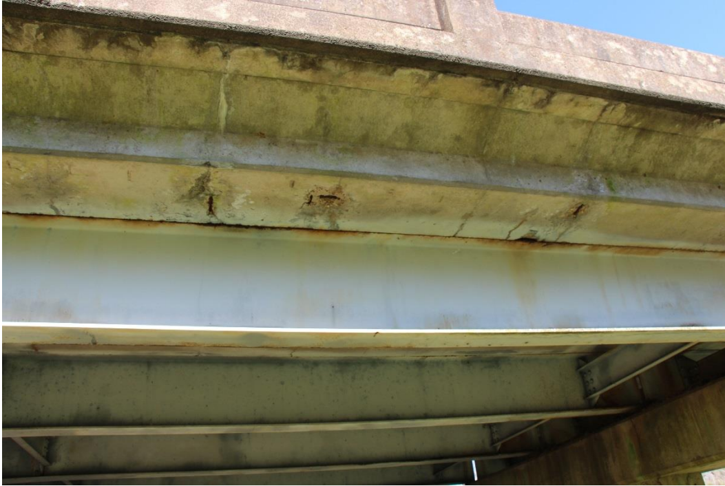
Condition Photo 7: Underside of the deck and curb, spalled with exposed reinforcing steel, typical.
