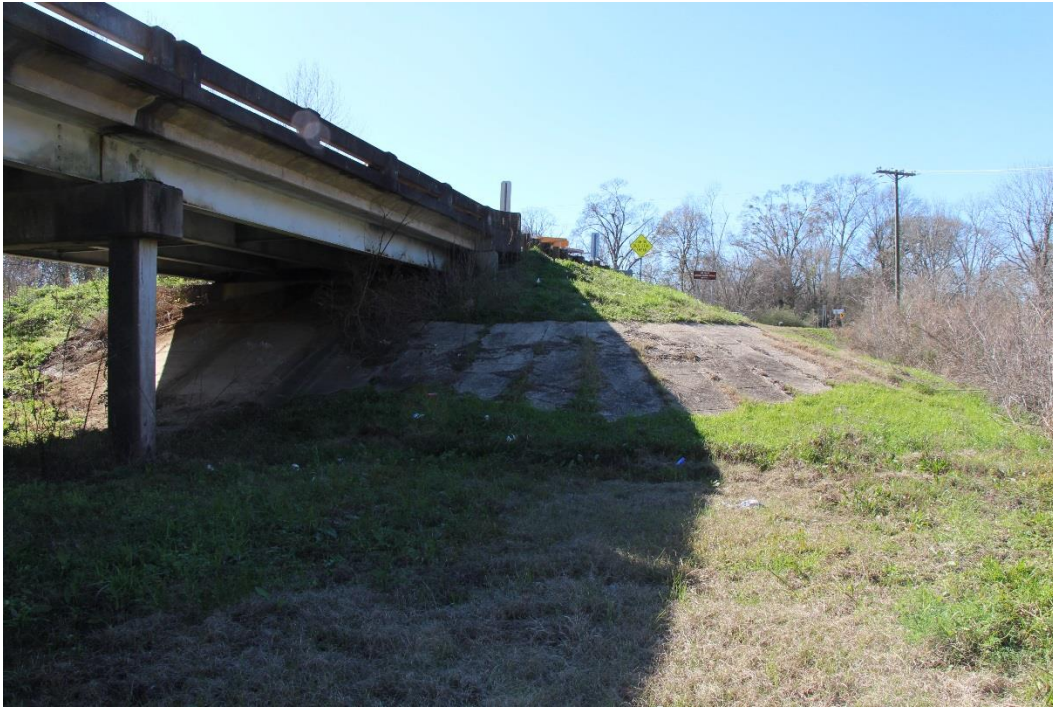
Condition Photo 17: Typical vegetation growth on the concrete slope protection at end bent 5.
