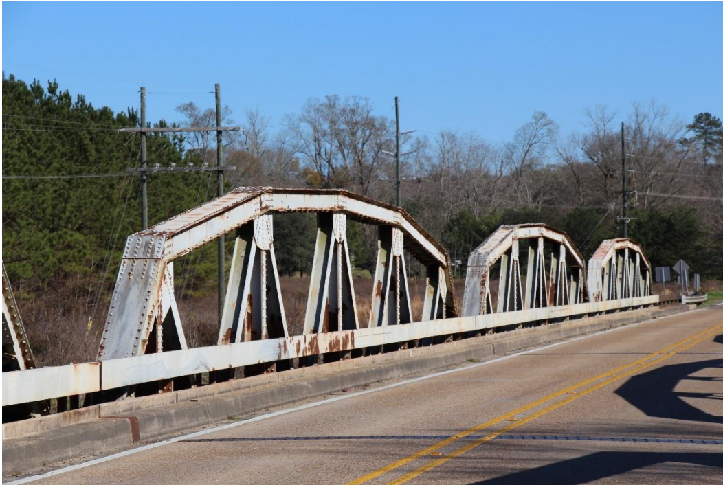
Character-defining Feature Photo 2: Design and construction of steel Warren truss spans. The Warren truss features diagonal members to withstand both tensile and compressive forces, added verticals for bracing, and a polygonal top chord.
