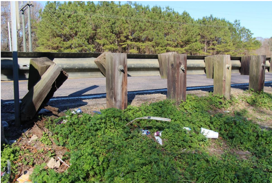
Condition Photo 18: Heavy decay to timber guardrail posts on the approach spans, typical.
