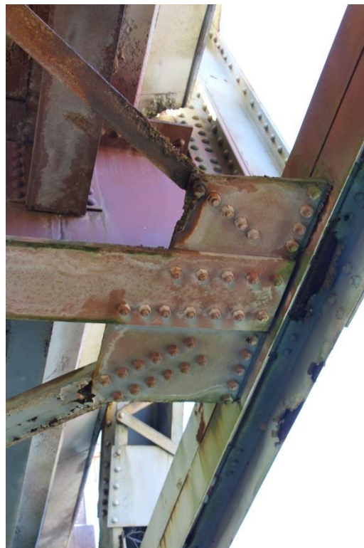
Condition Photo 12: Main truss span lateral brace connection rusted and section loss.
