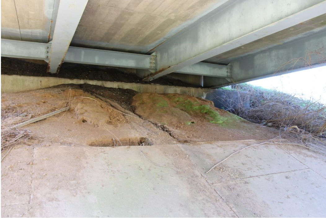
Condition Photo 15: Typical condition of end bent 5.
