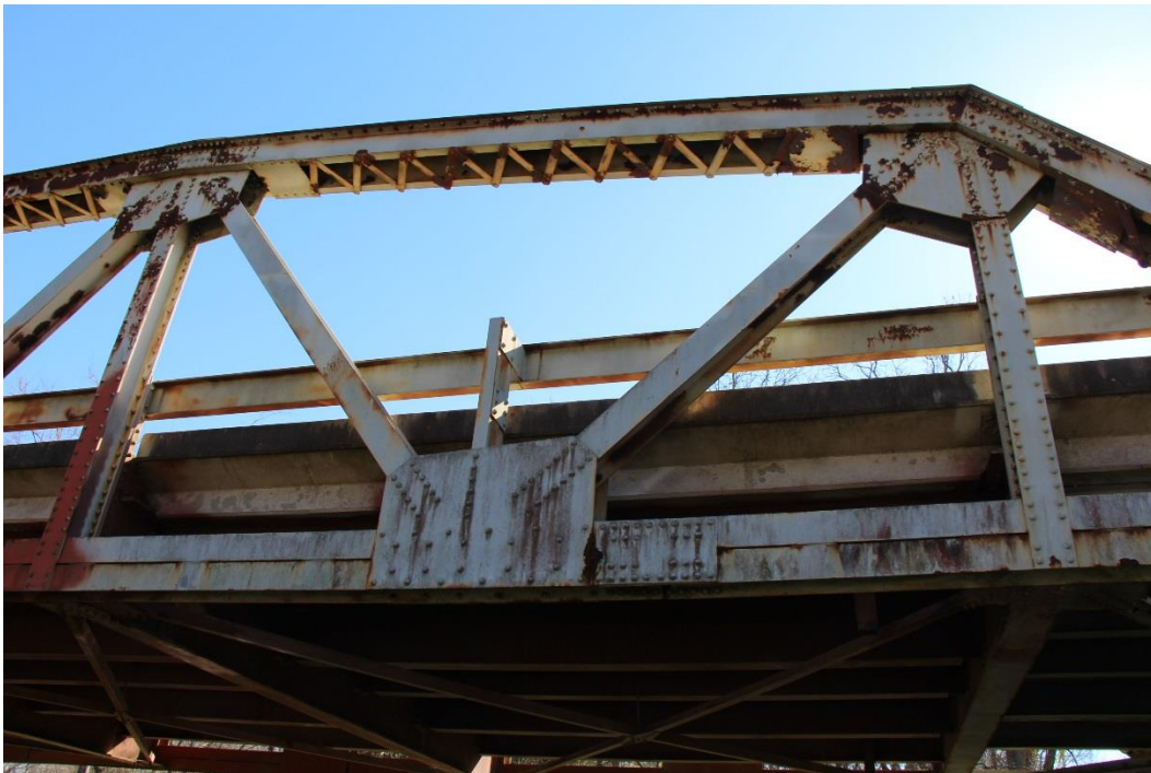
Condition Photo 10: Typical rust/corrosion and paint system failure on steel truss.
