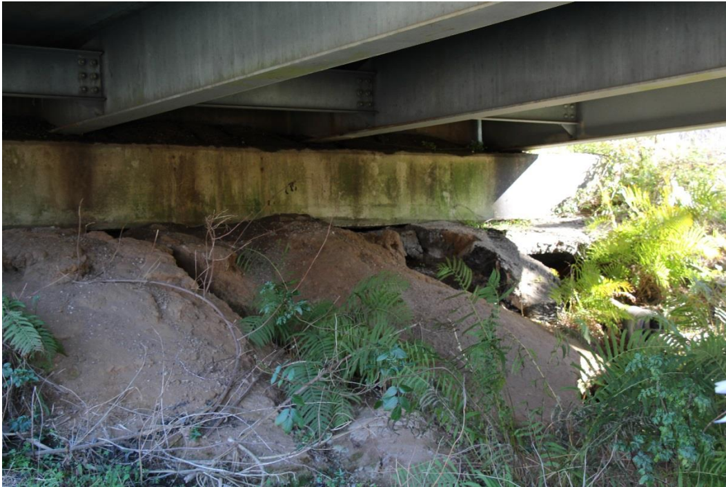
Condition Photo 13: Erosion at end bent 1.
