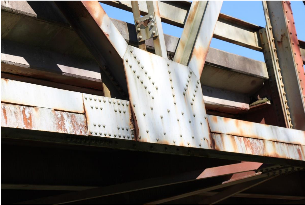
Condition Photo 9: Typical gusset plate connection exhibit paint system failure and corrosion.
