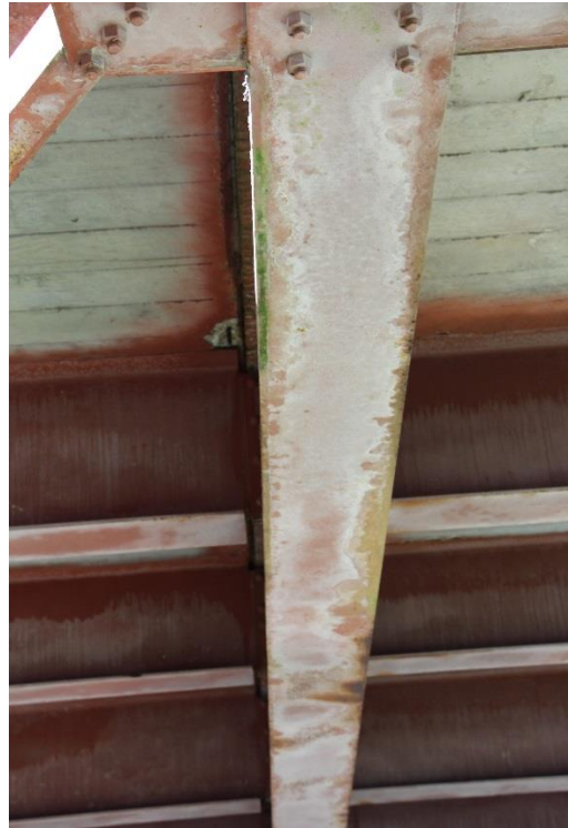
Condition Photo 11: Typical rust and paint system failure on the floorbeam.
