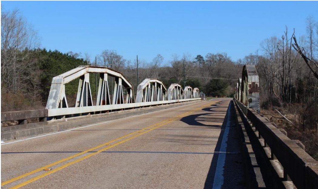
Condition Photo 1: Overview of the truss spans from the top of deck, looking east.
