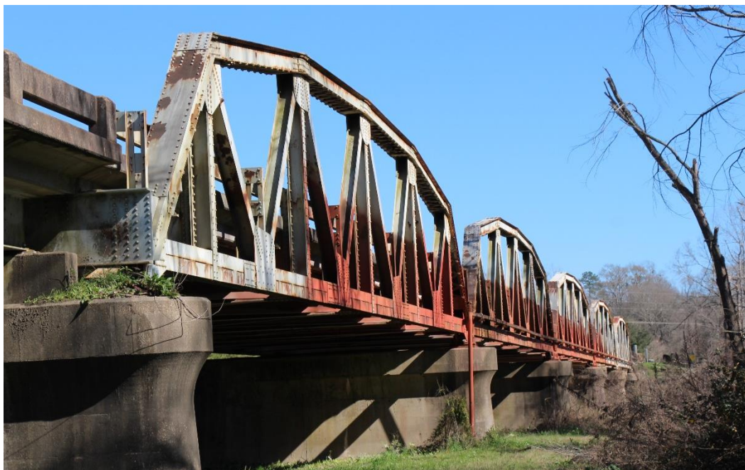
Character-defining Feature Photo 1: Design and construction of steel Warren truss spans. The Warren truss features diagonal members to withstand both tensile and compressive forces, added verticals for bracing, and a polygonal top chord.
