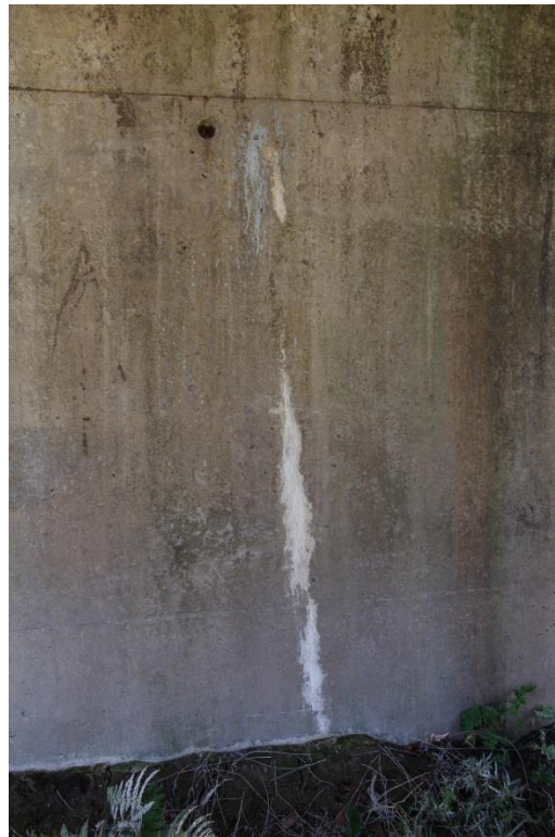
Condition Photo 16: Vertical crack end bent 5 seat with efflorescence.
